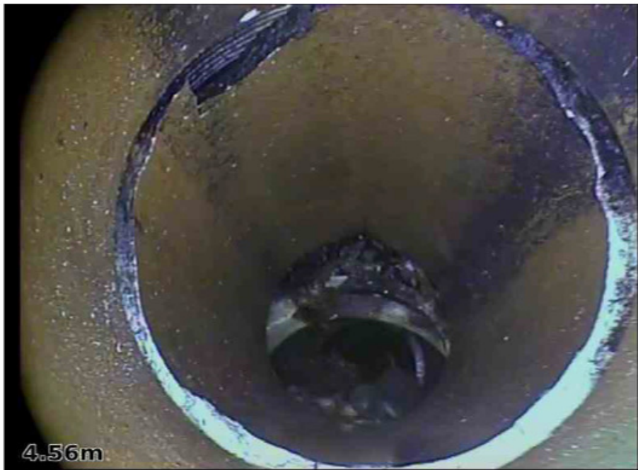
, 00:00:30, 4.56 m Broken pipe at joint from 10 o'clock to 11 o'clock
