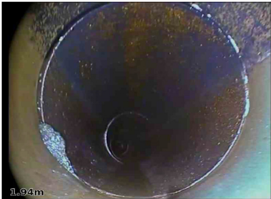
, 00:00:17, 1.94 m Settled deposits, hard or compacted at joint, 5% cross-sectional area loss
