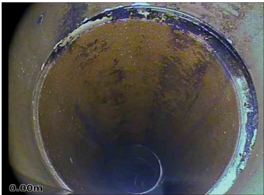
, 00:00:02, 0.00 m Open joint, large
