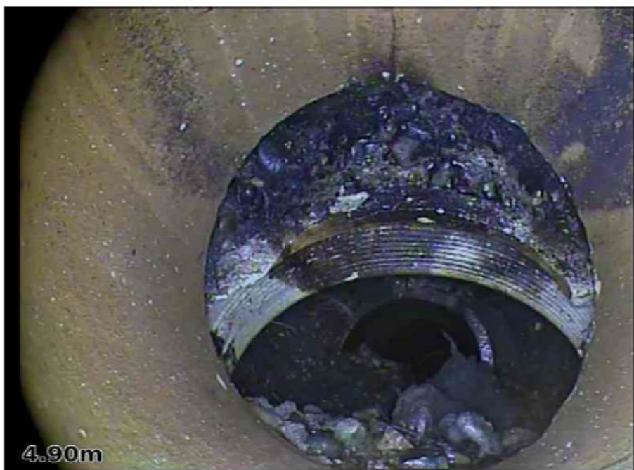
, 00:00:38, 4.90 m Collapsed drain or sewer
