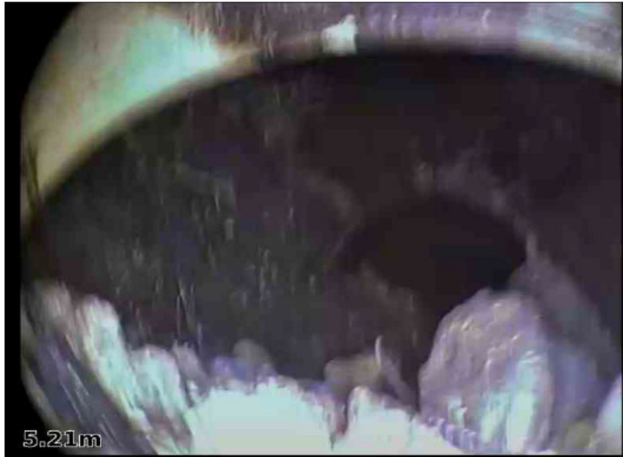
, 00:00:47, 5.21 m Survey abandoned, due to collapse
