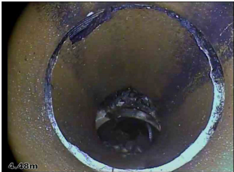
, 00:00:30, 4.48 m Open joint, large
