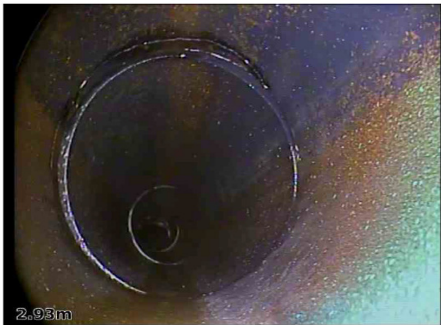
, 00:00:22, 2.93 m Crack, circumferential at joint from 9 o'clock to 1 o'clock
