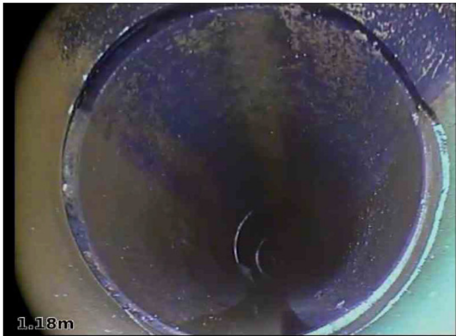
, 00:00:12, 1.18 m Crack, circumferential at joint from 2 o'clock to 6 o'clock
