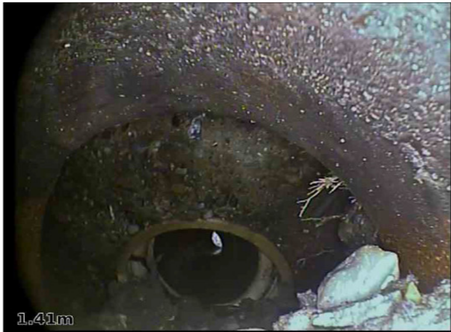
, 1.41 m Collapsed drain or sewer
