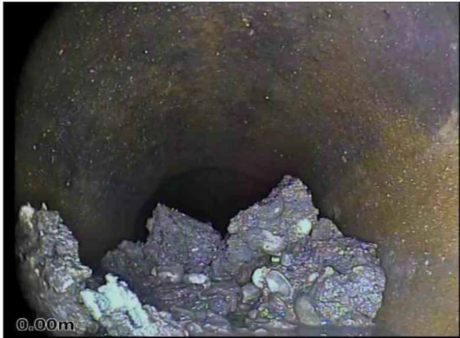
, 00:00:03, 0.00 m Settled deposits, coarse, 80% cross-sectional area loss
