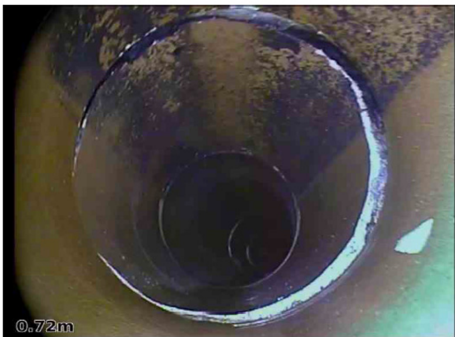
, 00:00:09, 0.72 m Open joint, large
